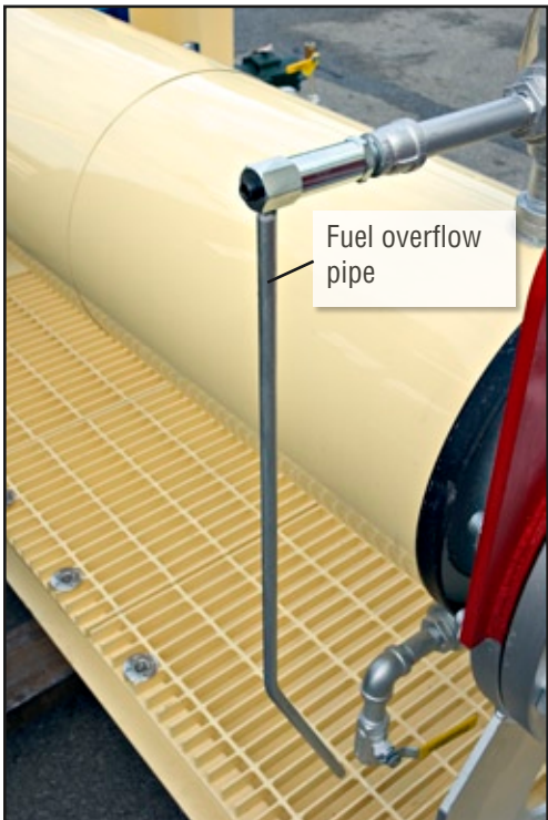
Figure 11. Fuel overflow pipe attached to the pressure relief valve on a skid-mounted preheater.
