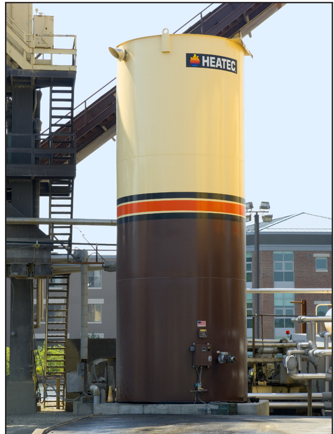
Figure 2. Heatec vertical fuel tank.
