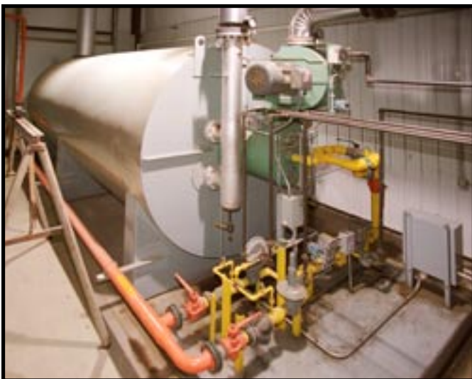
Heatec 21 million Btu/hour 3-pass heater at Froedtert Malt in Winona, MN.
